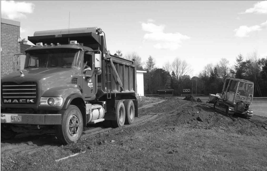
Haley Construction truck brings a load of fill from Hardwood Products construction site for placement around grade 7-8 wing at PCSS by Lemieux Construction.
