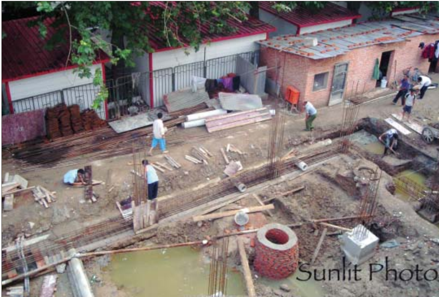
The humble beginnings of a new skyscraper in Beijing. Workers from the countryside live in the brick bunk houses and toil from sunup to sundown (often in flipflops) with simple tools. Photo by Jeanne Griffin.
